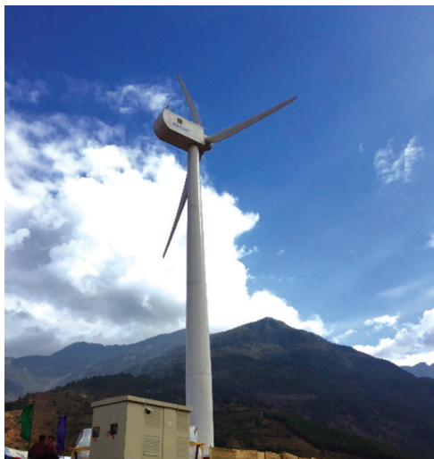
Figure 6 The 600kW Wind Power Plant at Rubesa, Wangdue
