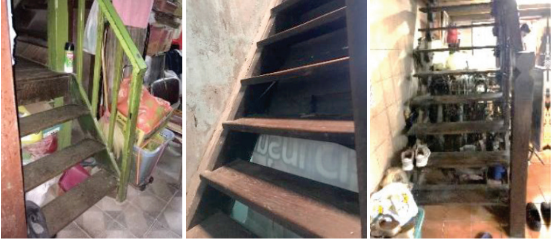
Figure 13. Inappropriate stairways found at the studied sites. (Sources: Photos taken by research team)
