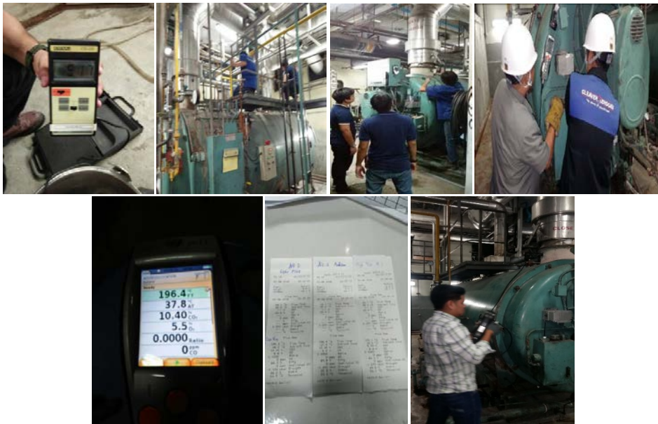
Figure 1 The measurement of boiler operations
