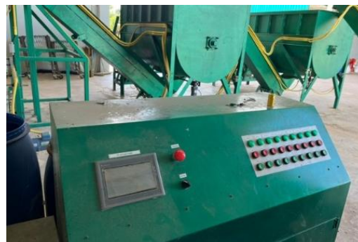
Figure 8 PLC-based electrical control cabinet.
