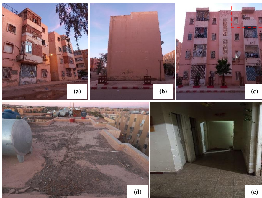
Figure 2 Actual photos of the studied apartment; (a) West facade; (b) South facade; (c) East facade showcasing the studied apartment framed; (d) Degraded flat roof (view from the North); (e) Inside the apartment
