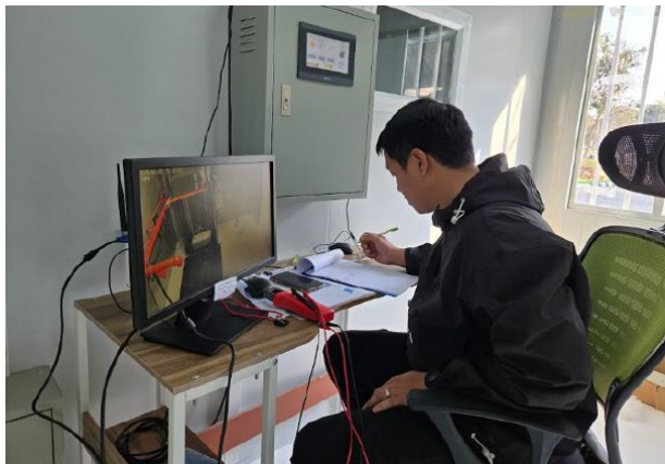
Figure 10: Control and observation room
