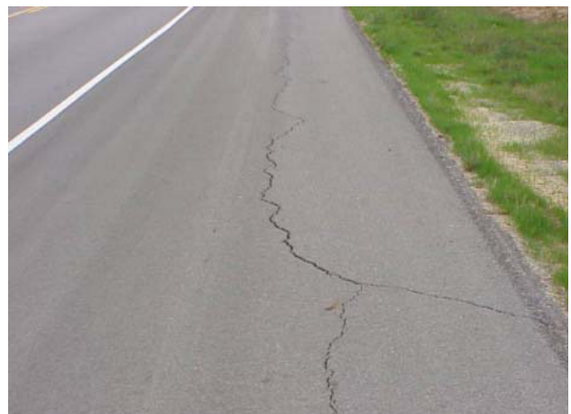
b) Pavement distresses from expansive soil movements
