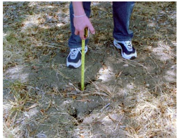
a) Measurement of desiccation crack in expansive soil area
