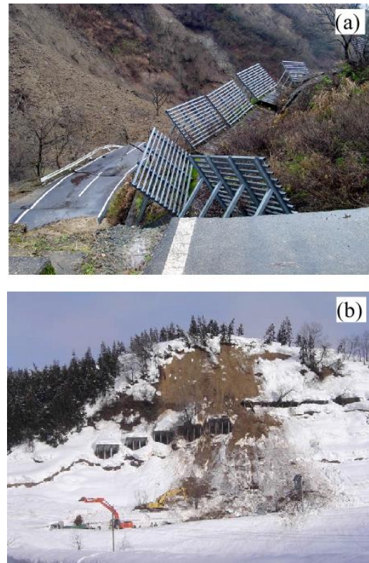
Photo 6 (a) Damage of snow avalanche fence and (b) a snow-earth avalanche (Kamiishi and Machida, 2008)
