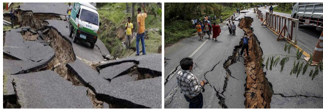
Figure 22 Damages of Transport system (mormonsoprano.com)
