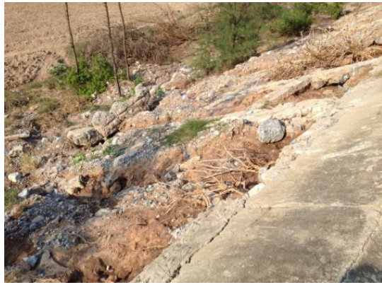
a) Destruction of outer slope by wave attacks, Thinh Long 22 Feb 2012
