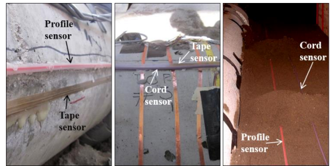
Figure 6 Example of sensors bonded to pipeline (left and middle) and being embedded in soil (right)
