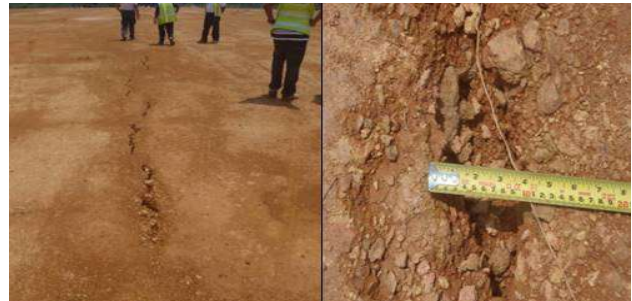
Figure 4 Longitudinal Crack found on the Embankment
