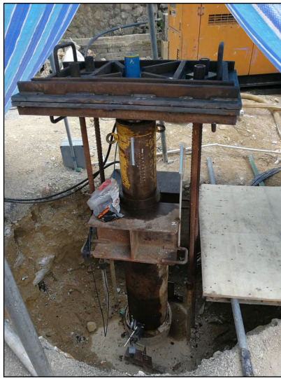
Figure 7 Setup at the site
