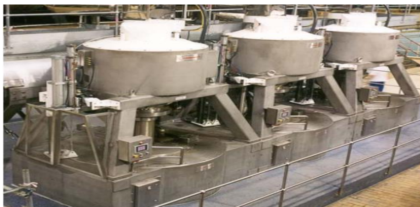
Figure 1 Battery of centrifugal Machine
