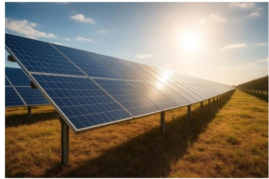
Fig. 1 Example of a fixed-tilt solar panel [22].
