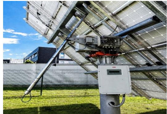
Fig. 2 Solar panel with a tracking system installed [23].
