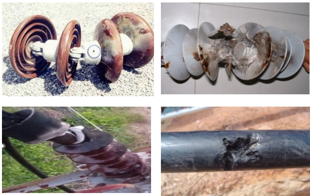
Fig. 1 (a) Suspension insulators damaged by arc burns, (b) Arrester explodes from overvoltage, (c) Voltage stress on the bushing, and (d) Damaged cable caused by flash overs.
